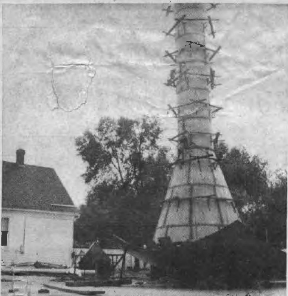
GOING UP behind the old Wheeling Village Hall on Milwaukee Avenue at Center Street is the new pedestal type water storage tank. Inclement weather, however, has delayed
